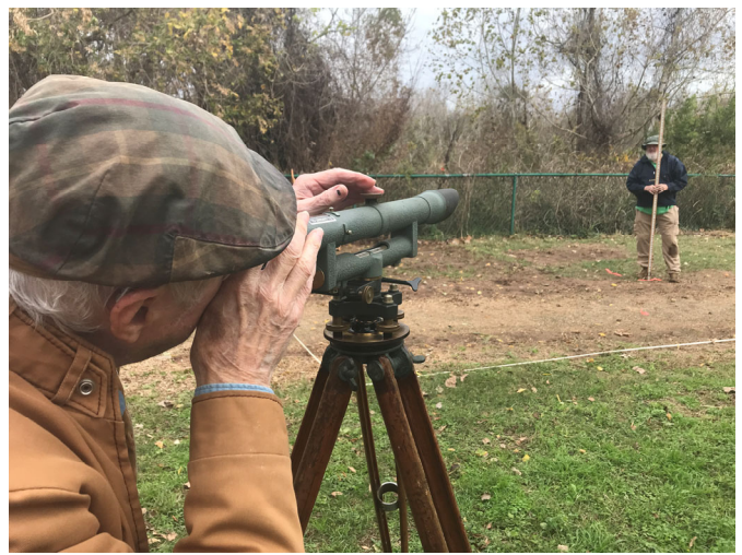
In addition to precisely establishing each corner of the new pits, the ground level at each pit is measured. This is done by comparing its elevation to a known point.
